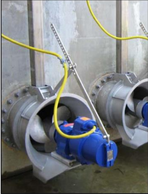
Figure 6-1 - Typical Installation of Flygt Mixer Pumps, Guard Rails, and Submersible Power Cable
