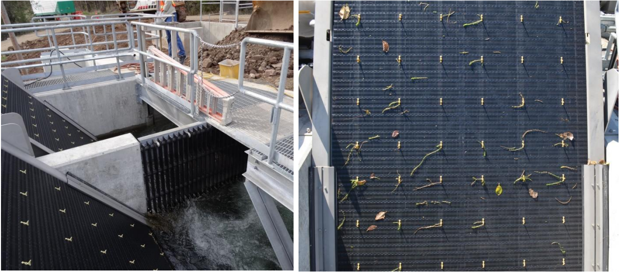
Figure 4-24 - Photos of the North Fork TSS Traveling Screens with Debris Pegs
