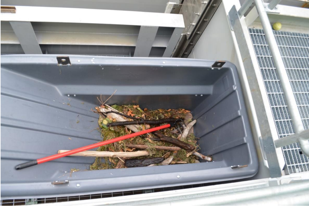
Figure 4-23 - Type of Debris Removed at the North Fork FSC Coarse Debris Rack
